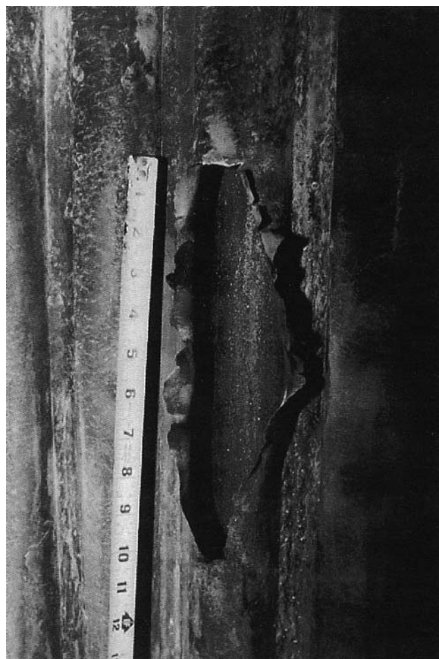
Figure 4 Waterwall tube failure in MSW incinerator.
