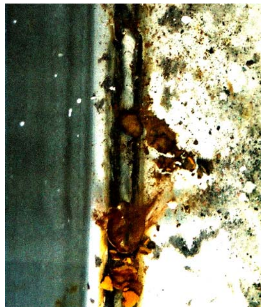
Figure 6: This weld within a swimming pool gutter was not cleaned properly and pitting corrosion is occurring along the weld seam. Photo courtesy of TMR Consulting
