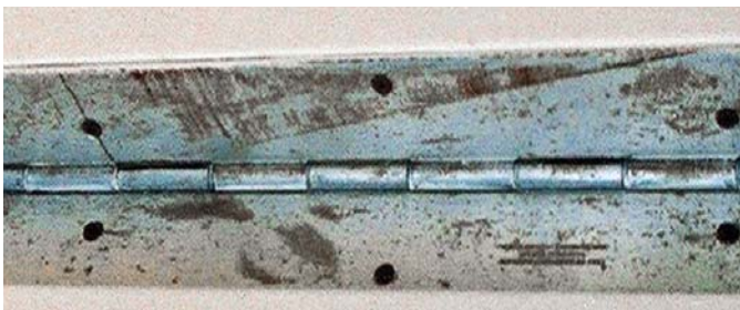
Figure 5: Carbon steel brushes were used by a cleaning contractor on this stainless steel door hinge that was installed beside an indoor swimming pool. The areas with carbon steel contamination are rusting. Photo courtesy of TMR Consulting
