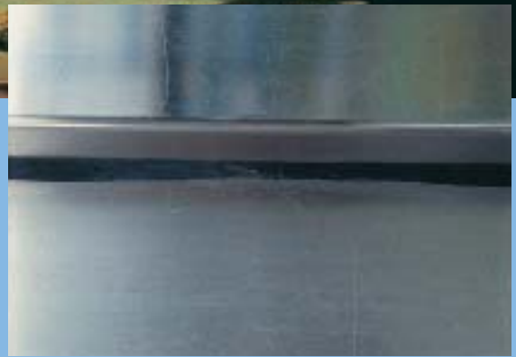
Stainless steel wall today
