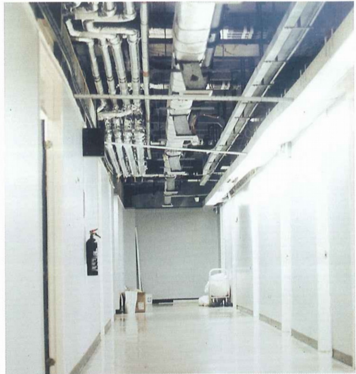
Stainless steel pipework in a hospital ceiling
