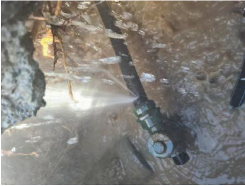
Image 1: typical failure of the Australian utility's PE-pipe.
