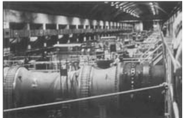
Figure 2 A gallery of laterals in the New York City pumping station. The laterals are made from cast stainless steel with 48 in. diameter wrought butterfly valves.
