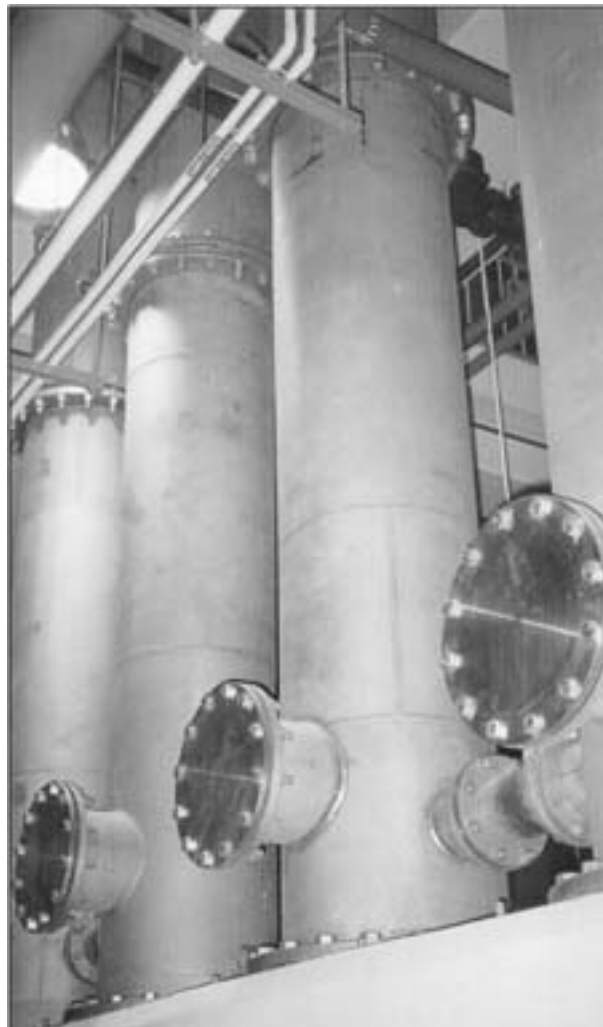
Figure 3 Typical stainless steel chlorine/ozone mixing towers
