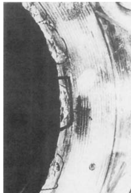
Figure No. 14 Closeup of flange in Figure 13 after cleaning. Shows open "gouging" corrosion that was directly under deposits.
