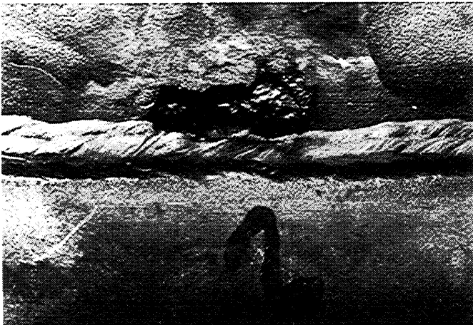
Figure 17 Attack in a field seam and immediately above it.
