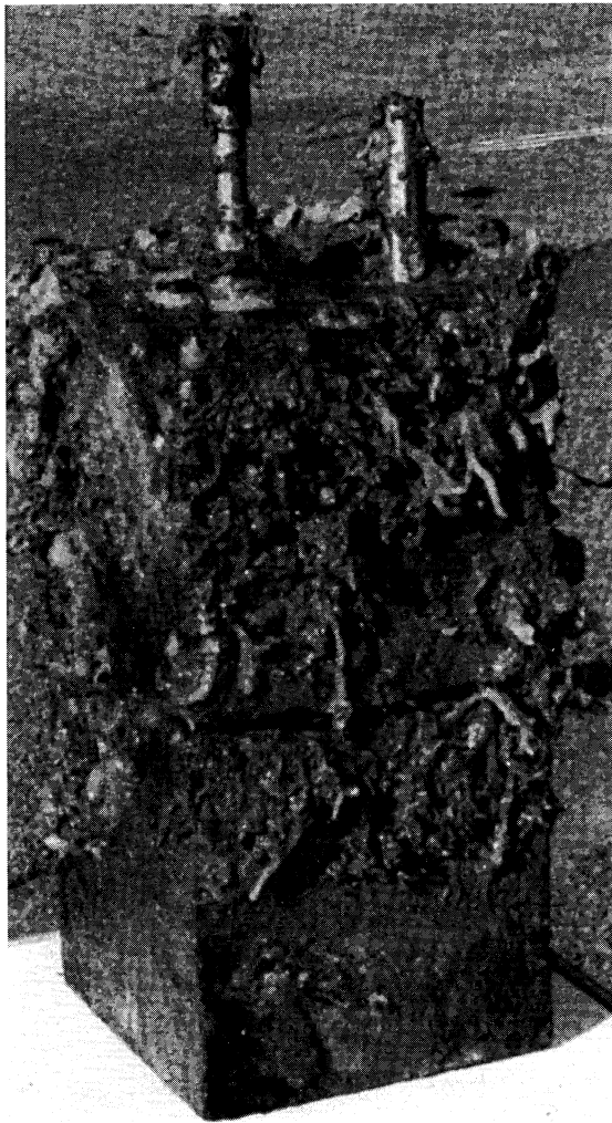
Figure 3: SRPC concrete blocks after 12½ years continuous exposure to seawater.
