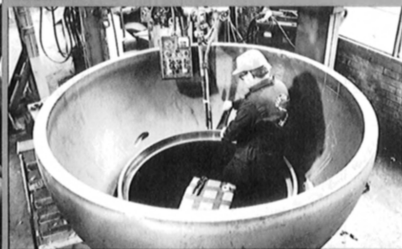
Figure 10—Shown here is a portion of the check valve, Figure 9, being submerged arc welded.
