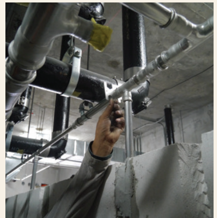
PHOTO STAINLESS STEEL PLUMBING SYSTEM
