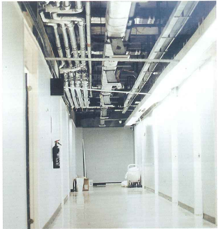
Stainless steel pipework in a hospital ceiling
