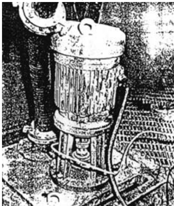
Fig. 13—Submerged pump handling 32% phosphoric acid–gypsum slurry at 170°F, from digester to filter. Submerged cast parts of ILLIUM "P"; shaft, bolts, nuts and studs are wrought Alloy 20.
