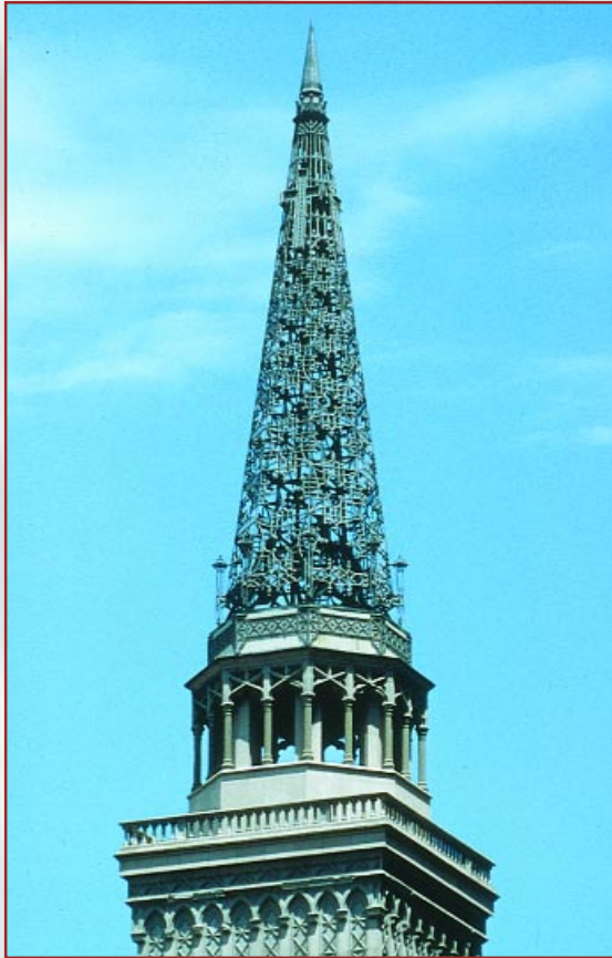
Smithfield United Church of Christ is a Historic Landmark built in 1926. The elaborate metal spire is aluminum castings on a steel structural frame. Both are painted. It was the first aluminum spire in the world. Architect: Henry Hornbostel.
