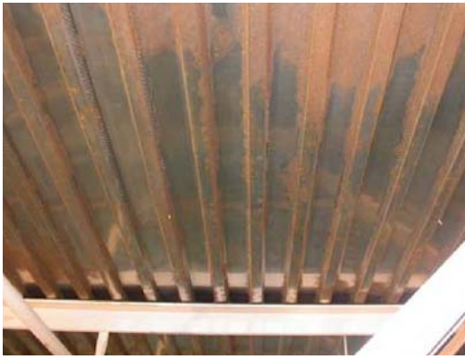
Figure 12: Corrosion of a Type 304 stainless steel roof deck above an indoor swimming pool. Photo courtesy TMR Consulting
