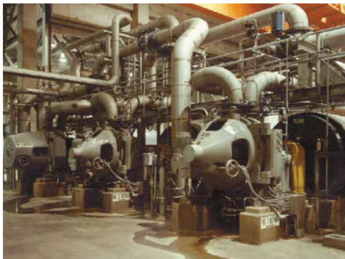
Figure 12-1 Refiner section leading to headbox approach piping
