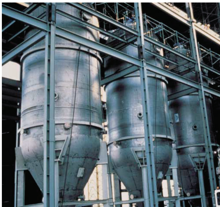
Figure 3-2 Alloy 2205 digesters at a mill in Thailand
