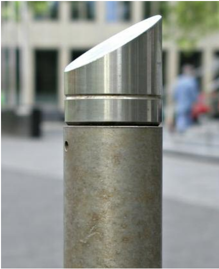
This Type 316 stainless steel bollard is exposed to road-salt splashing from passing cars. The bottom has a rough ground finish and the top a smoother polished finish which causes the performance difference. © IMOA
