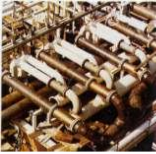
Figure 43. (DKI A 4974) Seawater cooling pipe system of CuNi10Fe1Mn (outside diameter 610 mm or 508 mm) for the TCP2 compression plant of "Frigg Field"
