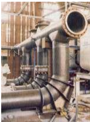
Figure 32. (DKI A 4971) Seawater piping system of CuNi10Fe1Mn on Texaco TARTAN A platform
