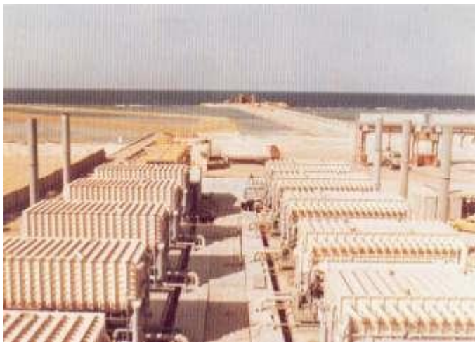
Figure 42. (DKI A 1226) Seawater desalination plant in Jeddah (Saudi Arabia) with an output of 10 x 500 m 3 = 5000 m 3 /day. All lines through which seawater passes, condensers, partition walls, tubes of final heater, housing, distillate troughs; and other important parts consist of CuNi10Fe1Mn
