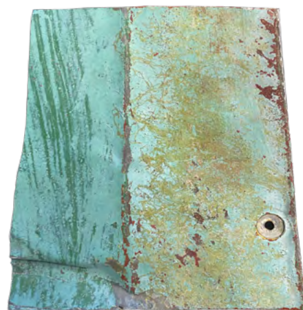
Battery maritime building Monel Side B
