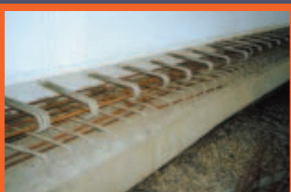
THE SIXTEEN PIERS of the Broadmeadow Bridge are reinforced with 169 tonnes of S31600 stainless steel.
