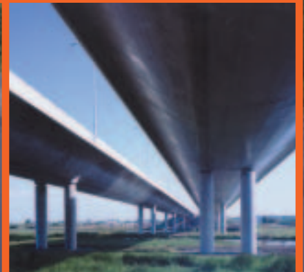
STAINLESS STEEL REBAR was essential to protect areas of the bridge which are vulnerable to corrosion from road salt.
