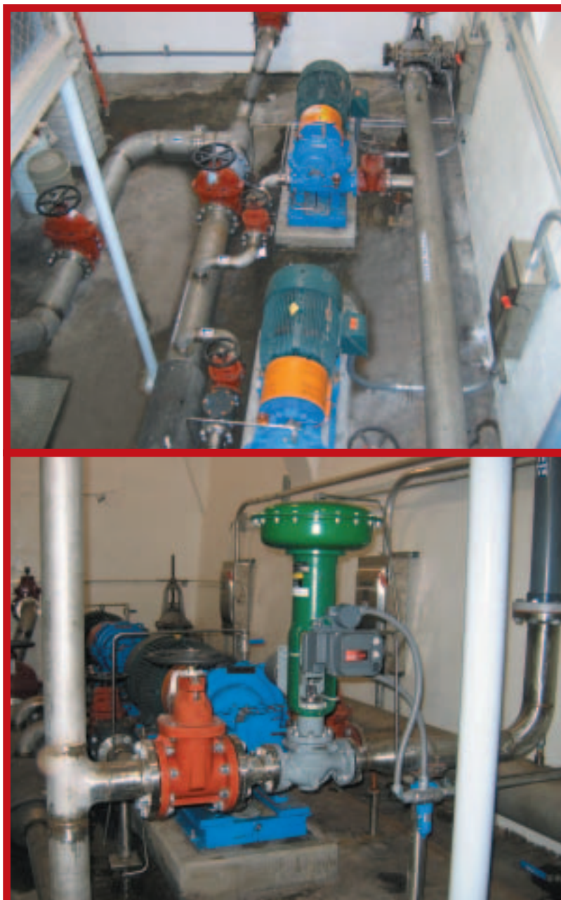
THE PIPING IN THIS WELLHOUSE on the University of Missouri’s campus in Columbia was replaced with S30400 stainless steel in 2004. Ease of installation reduced costs.
