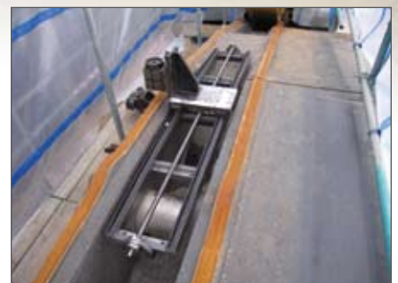
Rusted steel tracks with frame to hold milling machine
