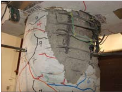
Severe damage in conventional steel and concrete column end
